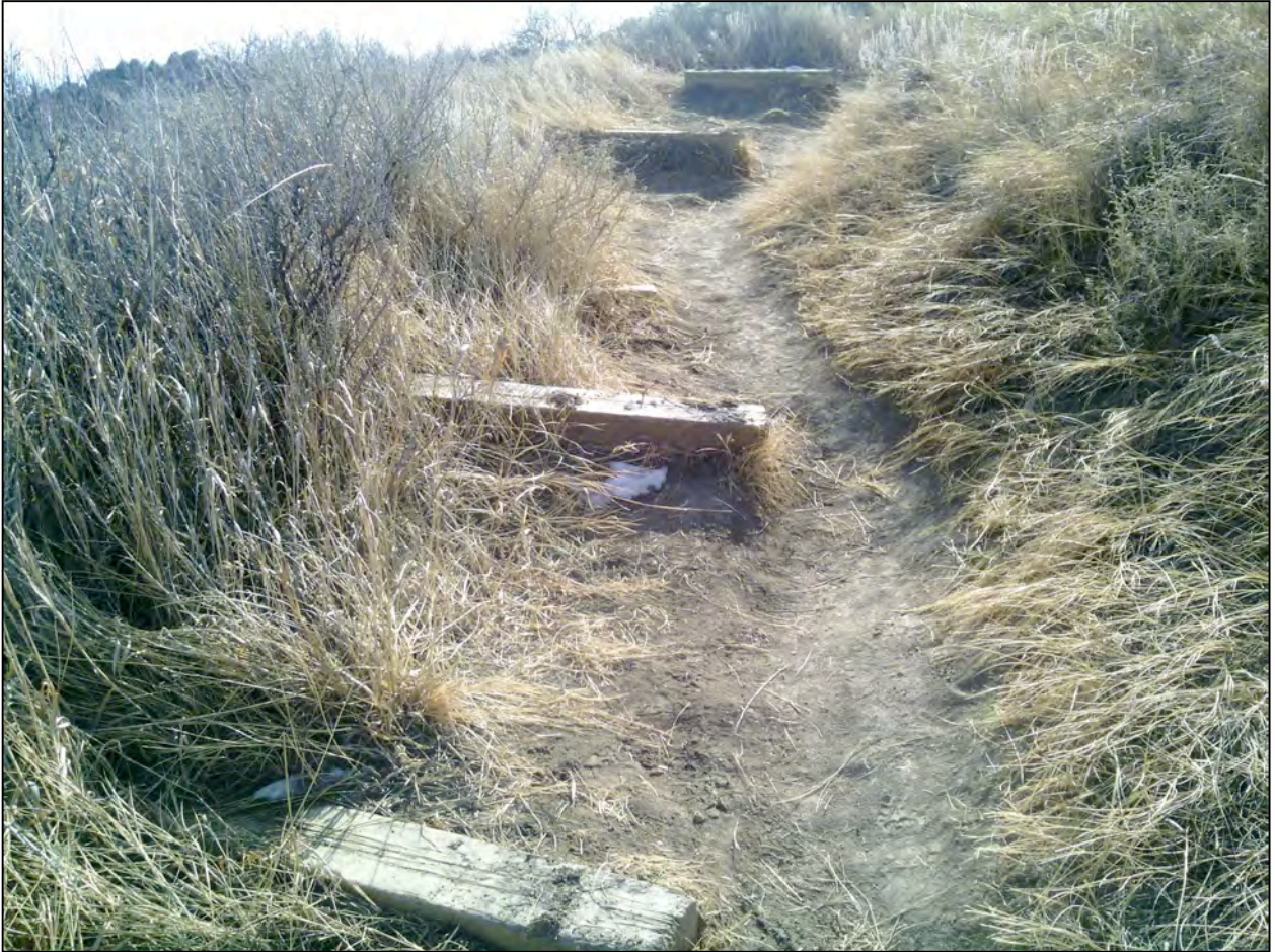
Figure 4. An example of a D-rated primary trail in the Garden of the Gods Park (Dakota Trail).
