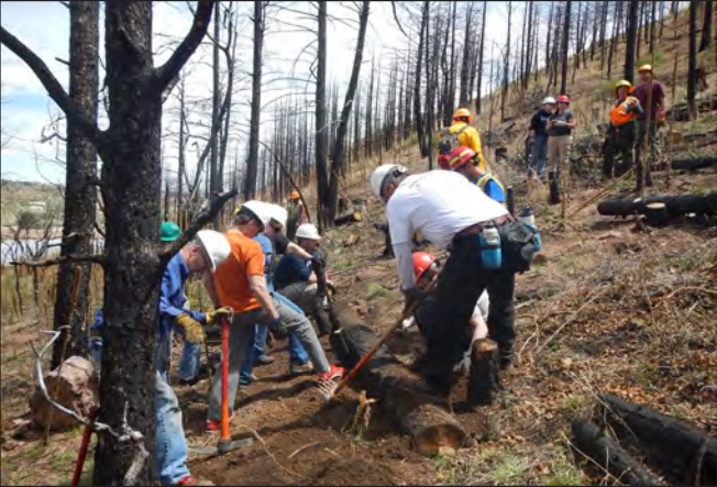
Participants in the annual Fire Restoration Skills Training learn from RMFI staff on proper construction of a log erosion barrier designed to stabilize hillslopes.
