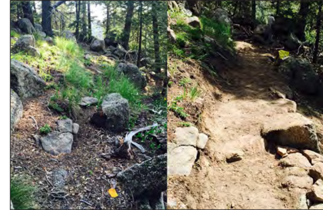
Before and after photos showing progress of new trail construction along the Top of the Mountain Trail in Cheyenne Mountain State Park.
