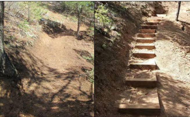
Before and after photos showing stabilization by timber steps along the new Mt. Muscoco Trail in North Cheyenne Cañon.
